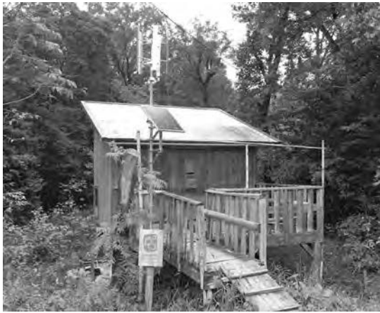
Figure 17. Solar panels and windpower generator (2016)
